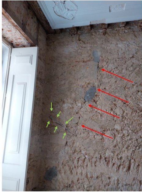
Figure 36 – Party wall showing a “Gato metálico” indicated by the green arrows and crack indicated by the red arrows. (picture taken on site and adapted for the case study)
