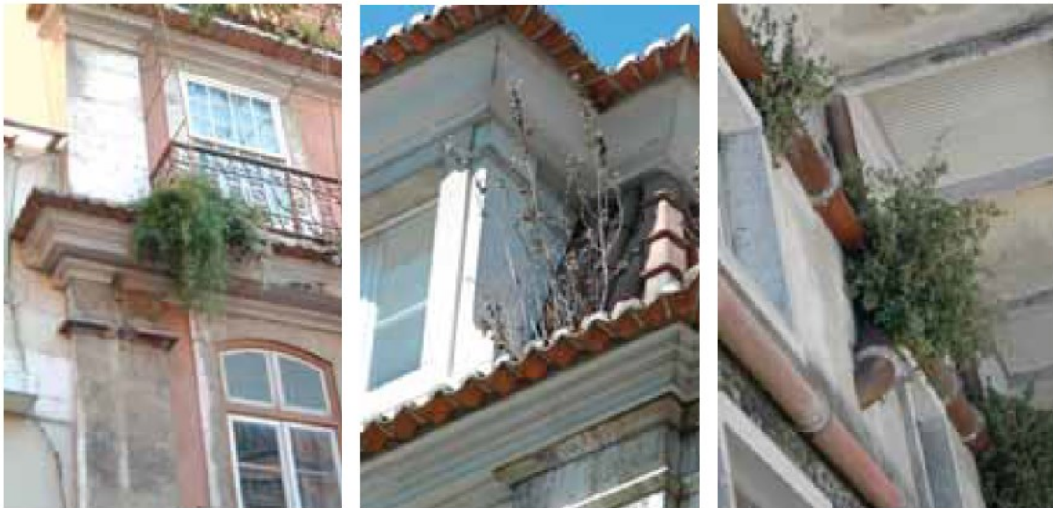
Figure 26 – Vegetation on facades which will cause cracking and detaching of elements (Lisboa, 2005)
