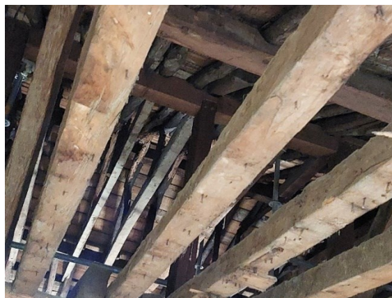
Figure 39 – Roof trusses, clearing showing burnt timbers that have been left in position ( Picture taken on site)
