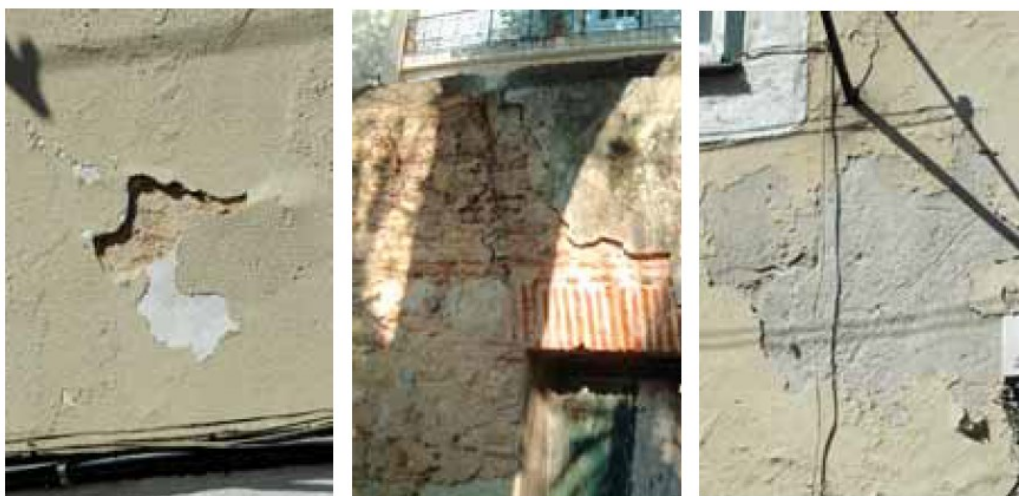
Figure 25 – Bad examples of rehabilitation with cementitious solutions which did not last long (Lisboa, 2005)
