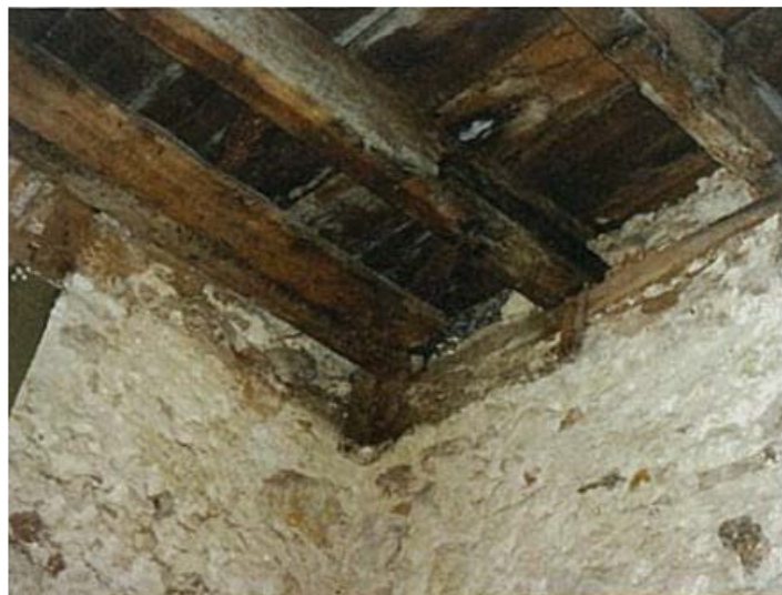
Figure 27 – Timber joists decay on its edges due to water ingress (Lisboa, 2005)
