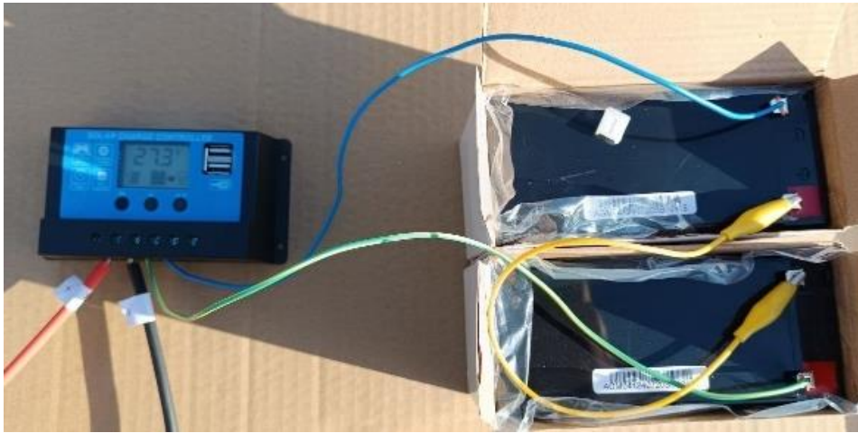
Figure 14 - Solar charge controller & Batteries
