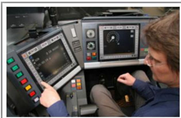
Figura 12. ERTMS – Cabine comboio [8]
