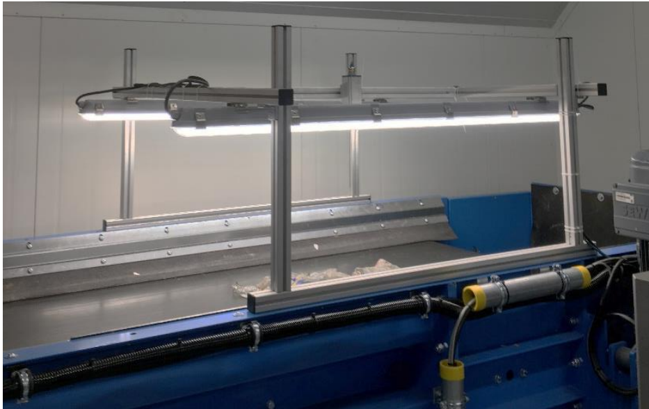
Image 1 – PolyPerception system installed in a plastic recycler.
