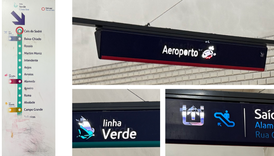
Figure D18: Aesthetic and technical problems with signage in the Lisbon metro. All photos taken by the author, 2025.
