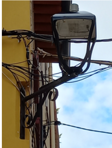
Figure 6.1: Luminaires and communication module
