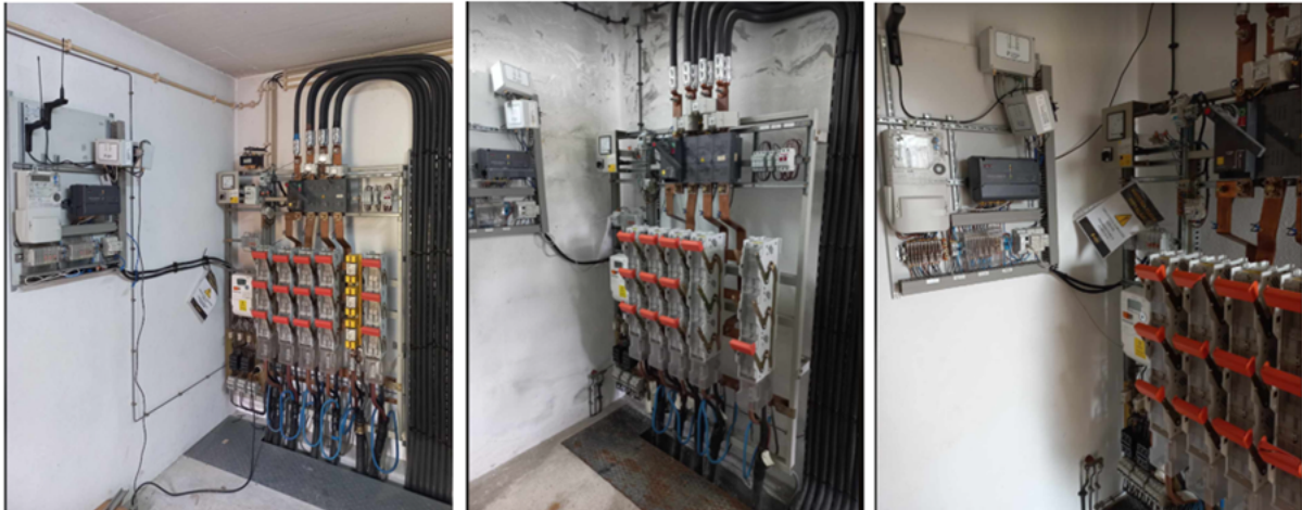
Figure 5.12: General low voltage panel a) 662; b) 663; c) 664
