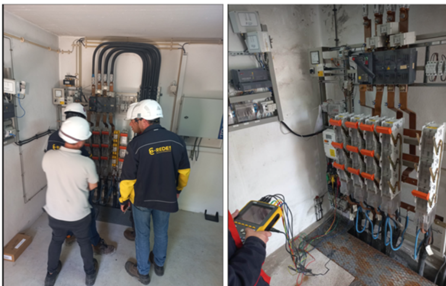
Figure 5.18: Installation of the energy analyser in TS
