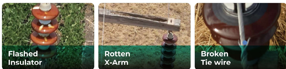
Figure 2.10: Examples of defects that are easier to detect during a virtual inspection [18]
