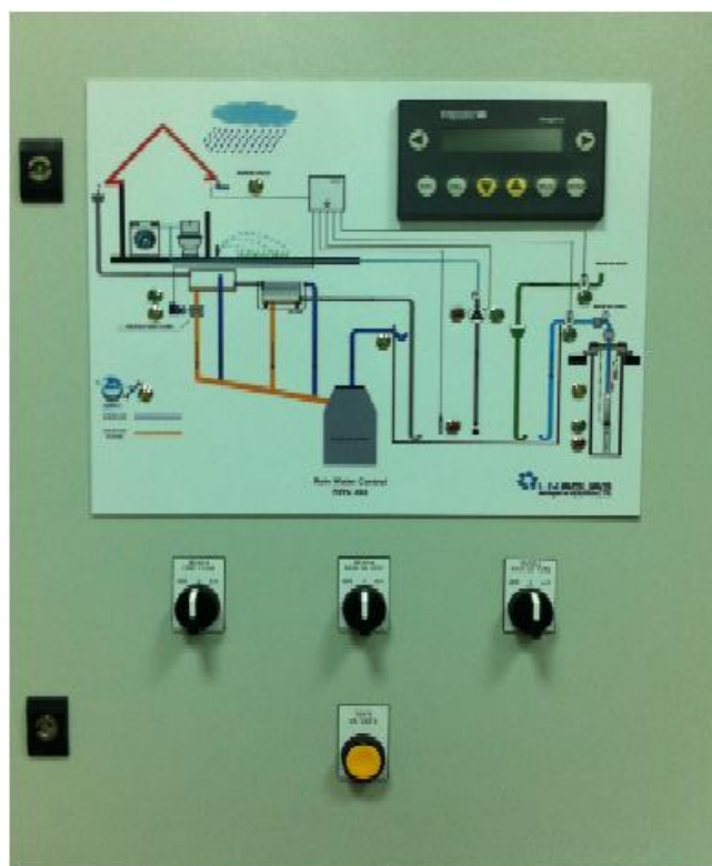
Figura 5.18 – Rain Water Control - RWC 303.
