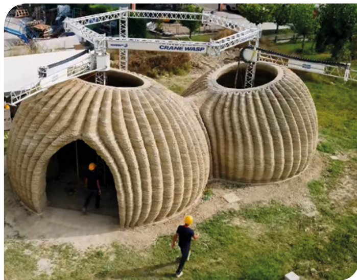
Figura 3 Construção sustentável com impressão em 3D (Vídeo Autor: Alfredo MilanoDrone views: ItaldronProject by:WASP: Engineering and 3D printing construction Mario Cucinella Architects: Architectural design and project managementIn collaboration with:SOS – School of Sustainability: Research partnerMapei: Materials consultancy and supplyMilan Ingegneria: Structural consultancyCapoferri: Frames engineering and productionRiceHouse: Bio-materials consultancy and supplyFrassinago: LandscapingLucifero's: Lighting designAriatta: Energy and internal comfort consultancyMola: Legno: Timber solutions consultancy and supplyPrimat • Terracuda@: Earthen floor supplyCefla: Electrical solutions supplyUnder the patronage of: Municipality of Massa Lombarda Sponsored by:Ter Costruzioni, CC BY 2.5 < https://creativecommons.org/licenses/by/2.5 >, através da wiki Wikimedia Commons).
