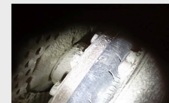
Damaged rubber coupling
