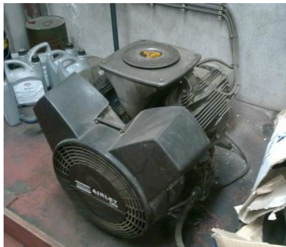
Figura 97 – Compressor Atlas Copco Airlet LE9.
