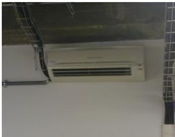
Figura 123 – Split mural da sala das UPS.
