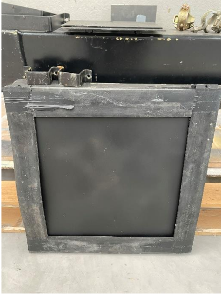
Figure 94: Inner ply completely intact after removal from the structure
