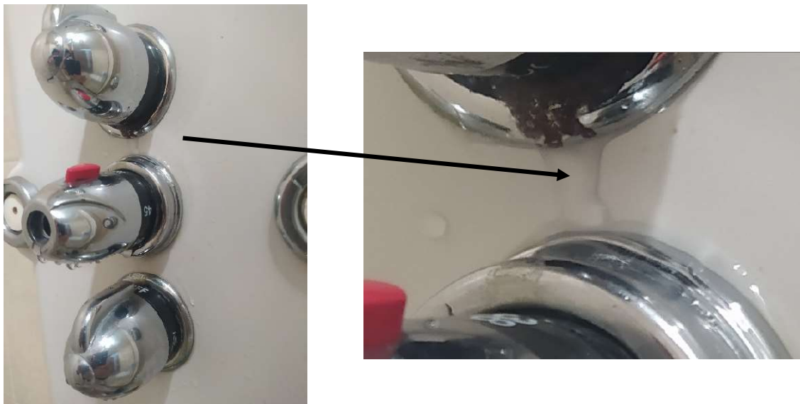
Figure 151 – Constant water leak of the shower faucet.
