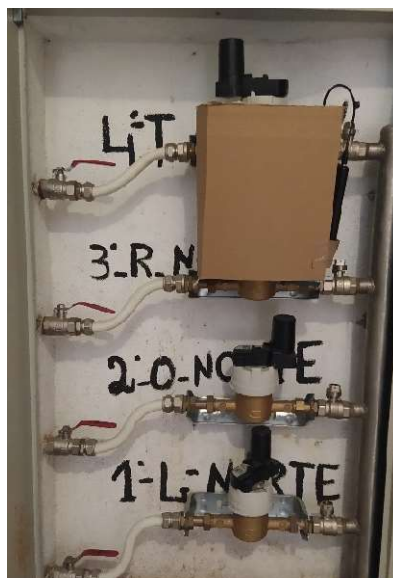
Figure 112 – Prototype placed on the water meter.
