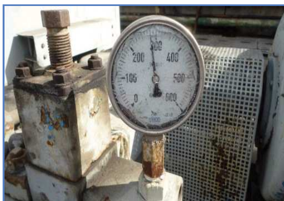
10 Pressure at pump outlet.
