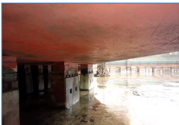
3 SBS-F.B. Condition prior to HPFWC.
