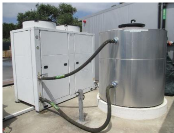
Figure 18 – Chiller in thermoregulation system.
