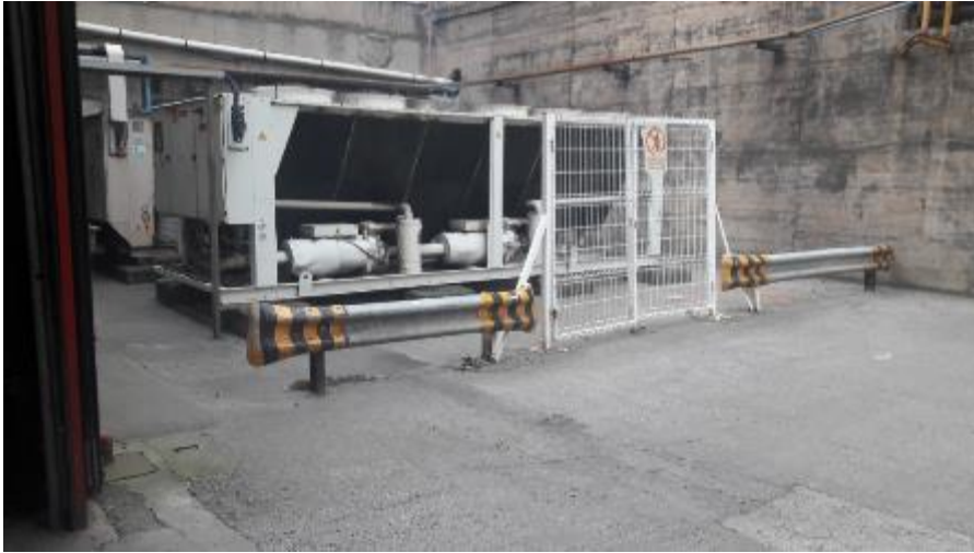
Figura 3.27 – Chiller Trane 1 e 2;
