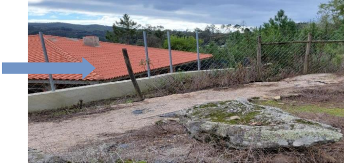
Figure 19 - Encroachment of Construction. Photo by Dan O'Brien 2022.
