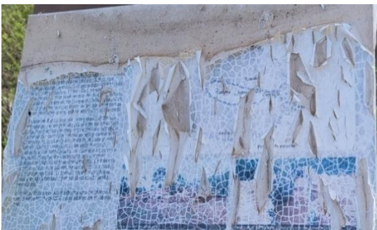
Figure 66- Sun damaged signage typical at Pozuelo Dolmens. Photos by Dan O'Brien 2022.
