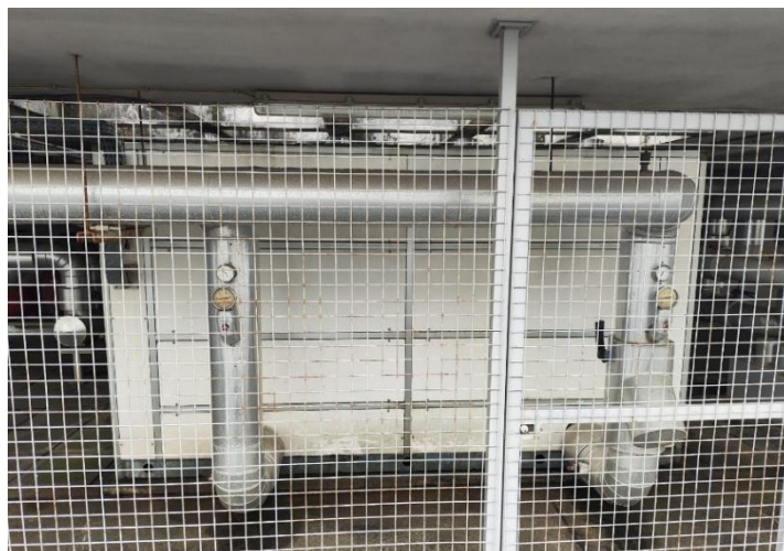
Figura 28 – Chiller RC Group UNICO A STD 142 F2
