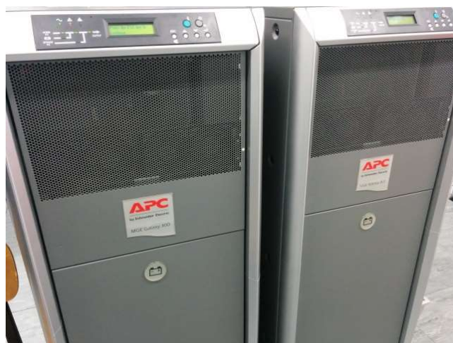
Figura 6- As UPS instaladas no DC
