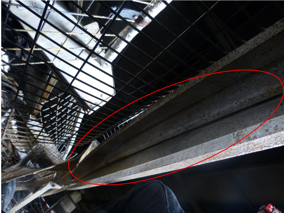
Picture 18 - View from underneath of metal bar on right side of previous picture – protected area (red ellipse), indicating fire did not come from underneath.
