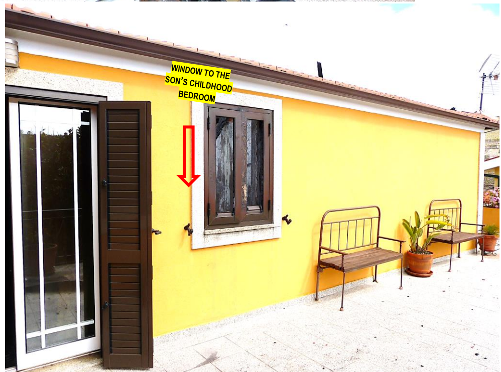
Picture 03 – View from outside of the window to the son’s childhood bedroom – damage with a propagation direction downwards (red arrow).
