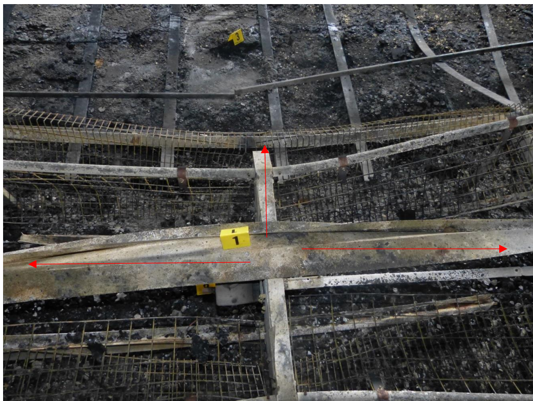
Picture 21 - View from top of tags #1-3, west (top) to east (bottom) – exposition levels on the metal bars are decreasing from tag #1 in the marked directions (red arrows); again, high deformation of metal bars shows exposition to high temperatures for a long time; high levels of carbonization on the floor (tag #3), indicating also a low level fires in that point.
