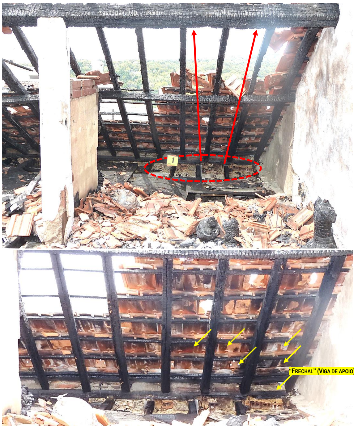
Picture 14 – By observation of the tiles, protected areas at the top can be observed –yellow arrows, compared to the side (surface) facing the floor, which has soot depositions from direct contact with the flames, confirming the upward direction of propagation of the fire as well as the development of combustion, with an increasing amplitude of the damage directly proportional to a point of origin on the bottom of the beam located on the main facade of the building – tag #1.
