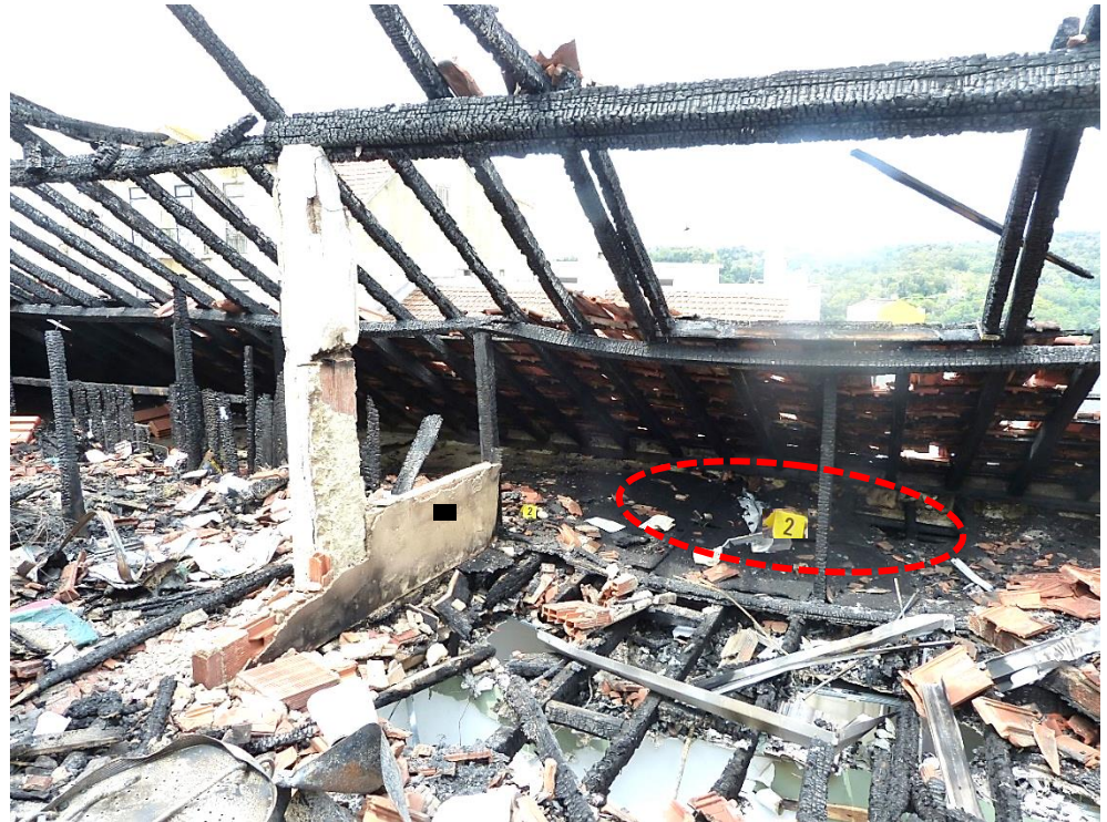
Picture 16 – In the adjacent space (towards facade on the left side) charring of the structure of the delimiting area was observed in an upward direction –red arrow- consistent with the incidence of a heat source- tag #2, which was close but at a lower level on the right side –red circle-.
