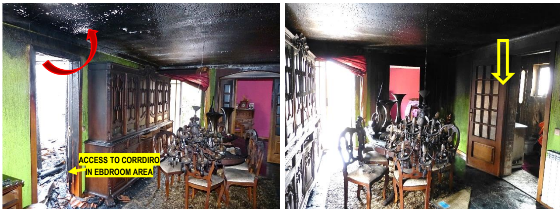
Picture 08 – General view of the dining room and access to the corridor leading to the bedroom area – damage observed on the ceiling – red arrow and in a downward direction - yellow arrow.
