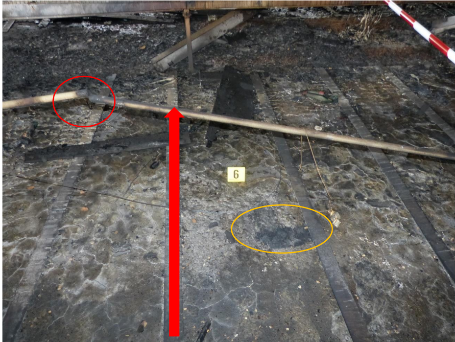
Picture 10 - Tag #6 – residues of detoxification blocs (orange ellipse), possible point of origin; high degree of carbonization and combustion can be observed on the floor, indicating a slowly progressed fire; red circle indicates the breaking point of the metal bars, indicating a long and high heat transfer in that point; the red arrow indicates on the metal bars on the floors an increasing damage and carbonization level from the bottom to the top of the picture (west to east).
