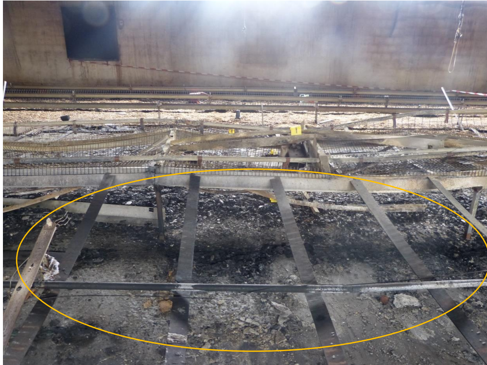
Picture 20 - View from east to west of tags #1-4 – metal bars are still in their original position, even though with levels of soot deposition and damage increasing from west to east; less damaged area than in the area behind (west) tag #1, indicating that the direction of travel of the fires was not towards this direction.
