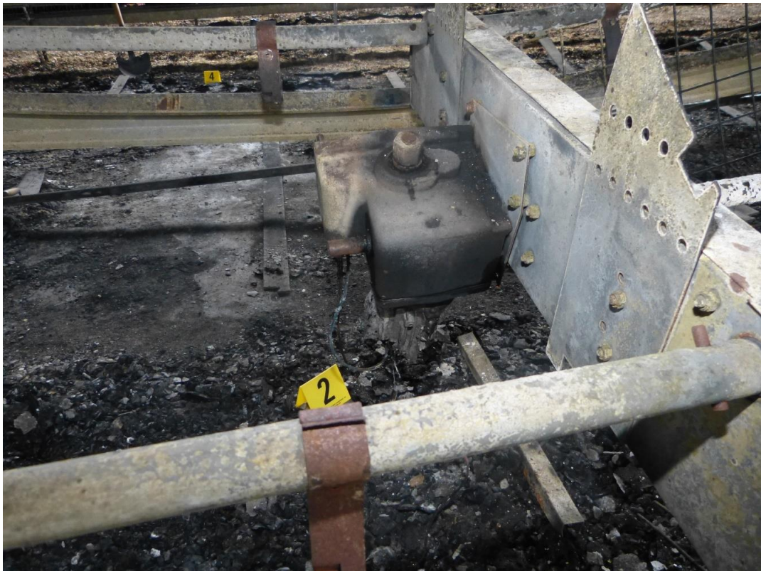
Picture 26 - View of motor (tag #1) from top, west (top) to east (bottom) – transversal metal bar area behind the motor shows signs of protection, but motor shows signs of heat transfer from underneath (black), indicating heat/fire source from underneath.
