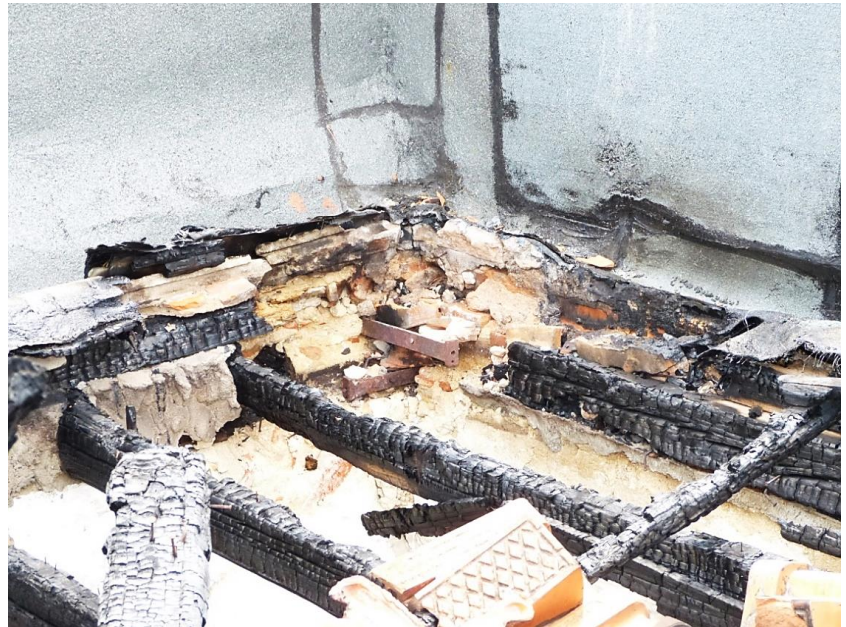
Picture 20 – Detailed view of the corner-area, where a heterogeneous damage in depth and downwards from the floor with a rounded shape is observed. This type of damage results from the combustion of fire accelerant in the initial phase, which was poured on the floor, allowing it to seep into the floor to develop a combustion at low level, in addition to allowing a spread in the initial phase of considerable intensity due to the evaporation capacity of the material used. It can also be observed that the combustion started in an area above the floor and below the roof structure, since a reduced damage of the sealing material of the curbs can be seen. The total combustion of the pavement in a circumscribed area downwards would lead to the partial destruction of the ceiling of the dining room in the lower floor, located right below the ignition point (see pictures 07 and 08).
