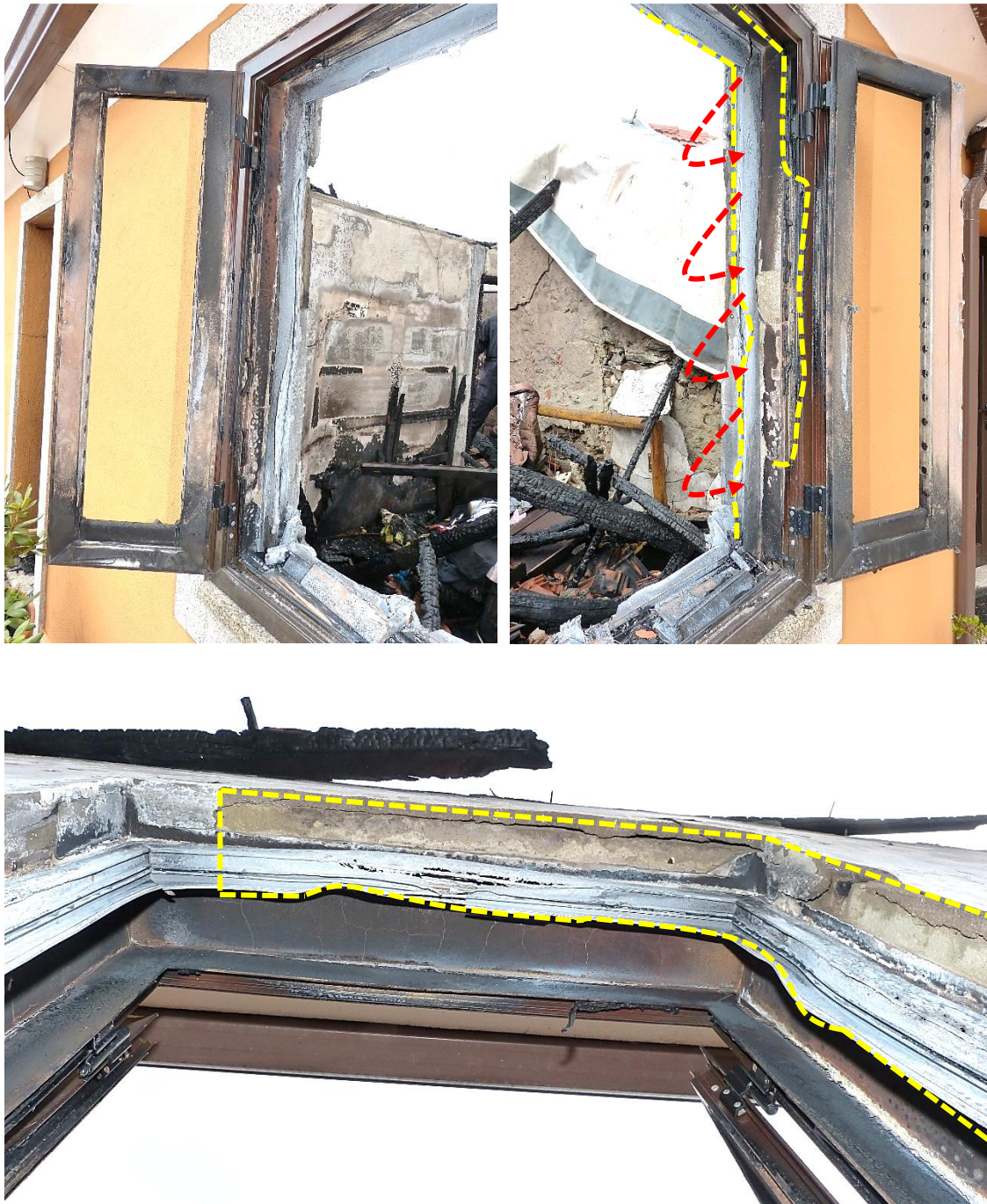
Picture 06 – The master bedroom window shows, albeit to a lesser extent, a higher concentration of the damage on the right side of the aluminum frames –yellow frame-, in line with the incidence of a low heat source with intensity but slowly – red arrows - from a point below and located on that side.
