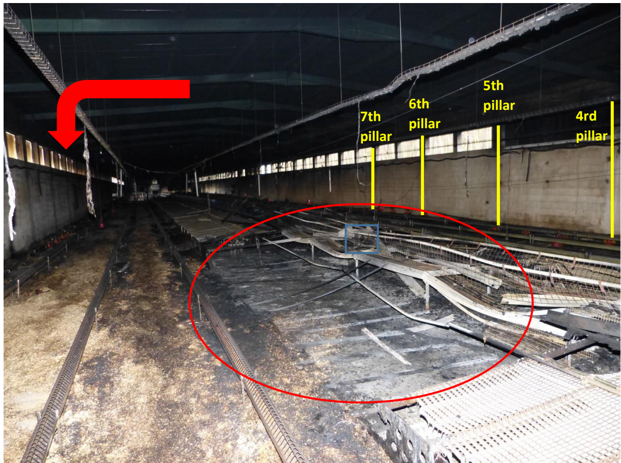
Picture 04 - First major damage area between pillars 3-7– View from left side (west) of the pavilion; the red circle indicates the area with the highest degree of damage, due to the complete absence of the covering fences, high carbonization level of the material and high soot deposition, also the metal bars are highly bent, which indicates a longer persistence of the flames in that area, which is an indication of a slow developing fire; additionally, major damage and soot deposition can be seen on the ceiling and from there the soot deposition level decreases from the middle to the outer part of the building as well as from the upper part of the walls going down, indicating that the fire propagated from the inside towards the outside and that the flames went up in the middle and then were deviated to the sides once they reached the ceiling, which is a typical phenomenon observed in compartment fires; also, one possible point of origin can be the blue squared engine, where the most damage can be seen.
