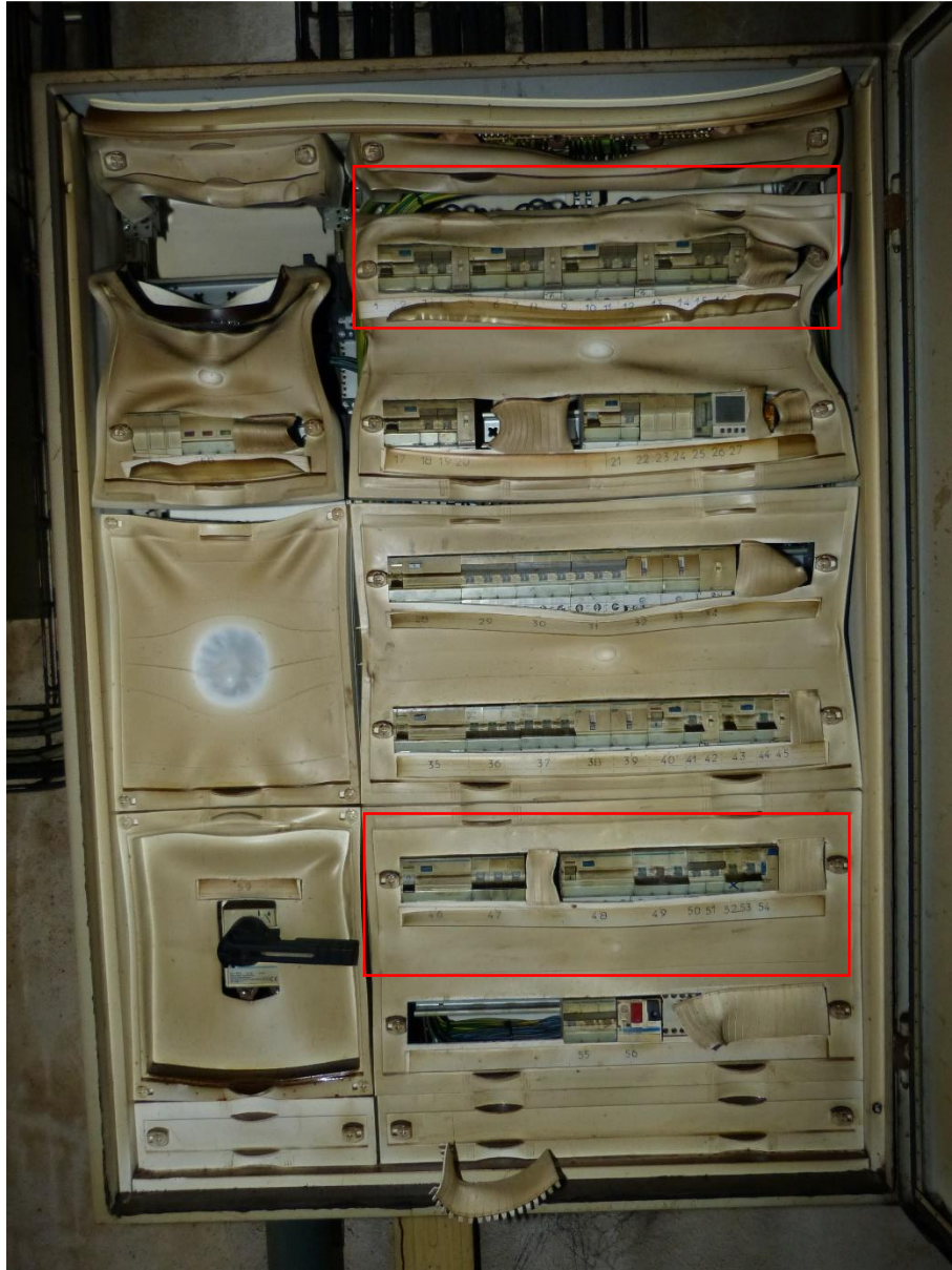
Picture 46 - Electrical box – red rectangles mark the areas repaired by the electrician.
