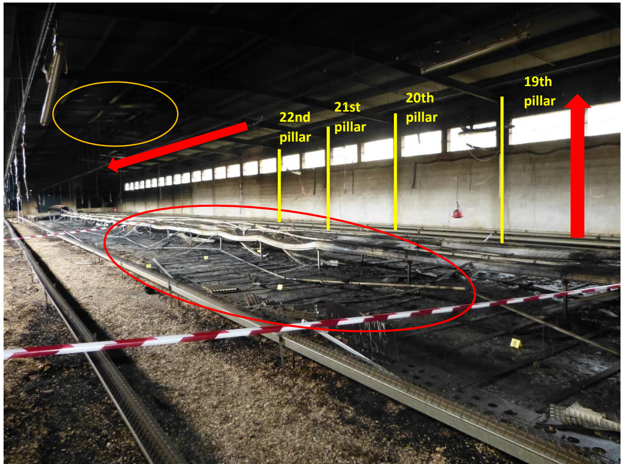
Picture 09 - Rear part of the pavilion – view from south to north, second area with major damage and possible location of second seat of fire; more extensive damage to the chicken-houses, since most of the roofs are completely destroyed, high level of carbonization; high deformation degree of the metal bars and soot deposition and oxidation signs (red ellipse), signs of a long persisting fire in that area, with the fire going upwards – convective heat signs on ceiling – and then from the middle outwards towards the walls; orange circle shows signs of higher degree of damage on the ceiling, indicating direct flame contact and for a longer period of time in that point; also, the deformation of the light bulbs shows signs of radiant heat.
