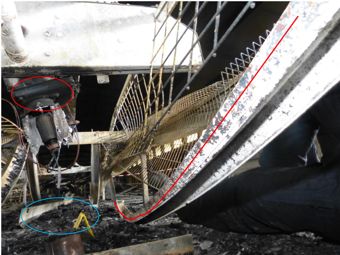
Picture 17 - Tag #2 – view from the left side (north to south) – metal bar on right of picture shows strong deformation in front of the motor and increasing oxidation from north to south – also, dropdown from melted plastic of bottom motor part – black underneath motor (red ellipse): radiant heat from second fire (blue ellipse).
