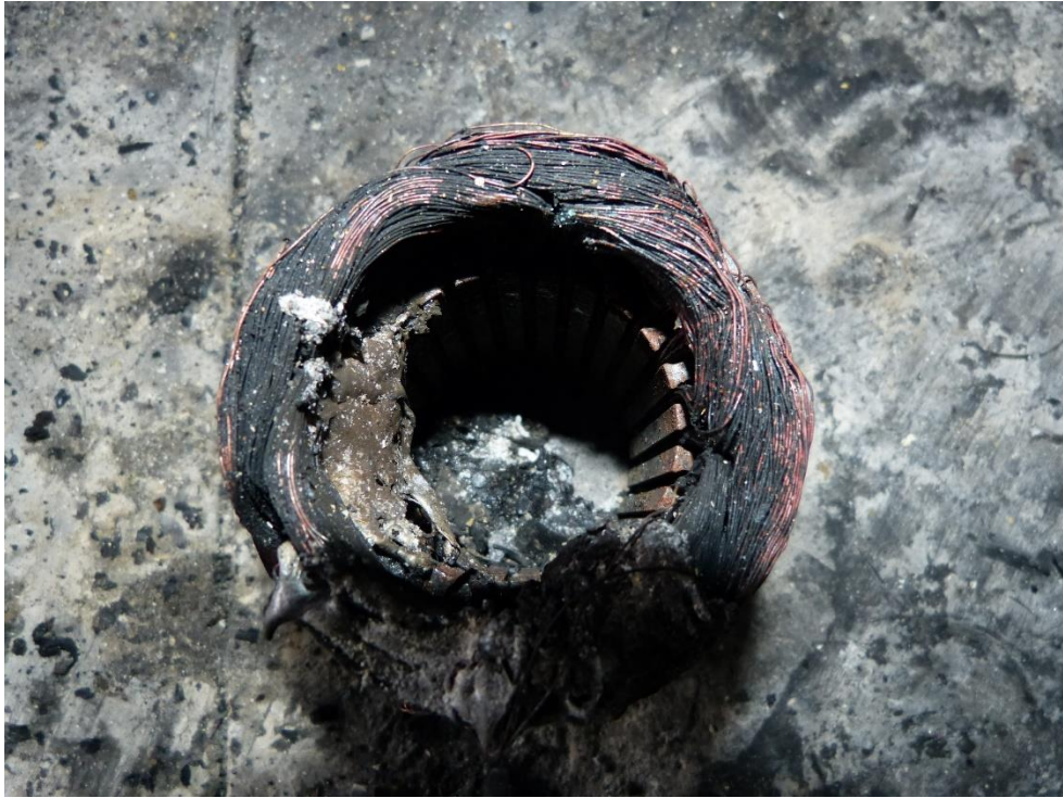
Picture 31 - View from top of part of motor (tag#1) that dropped to floor.
