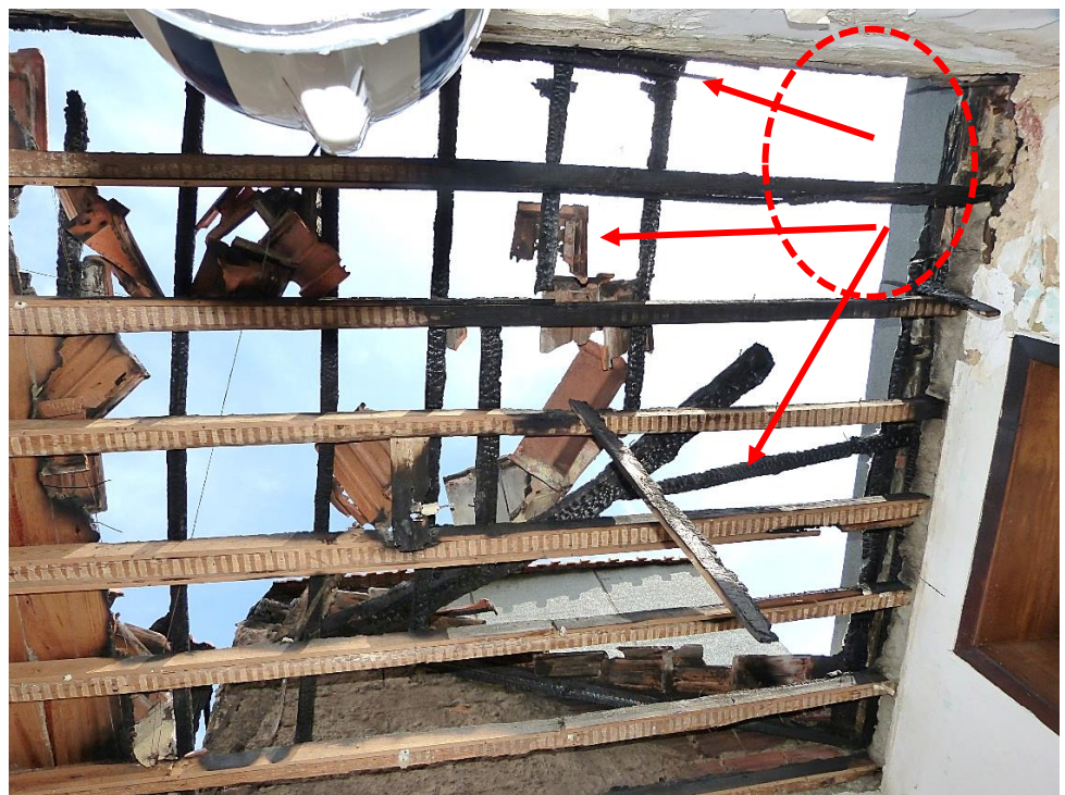
Picture 06 – In the roof area it is possible to observe a converging carbonization area along the support beams near the corner -red circle-, which results from the proximity to a point of origin. The absence of a greater extent of damage throughout the room, in particular by soot-fixation, arises from the rupture of the ceiling, which allowed the smoke of a small secondary fire outbreak to exit upwards.
