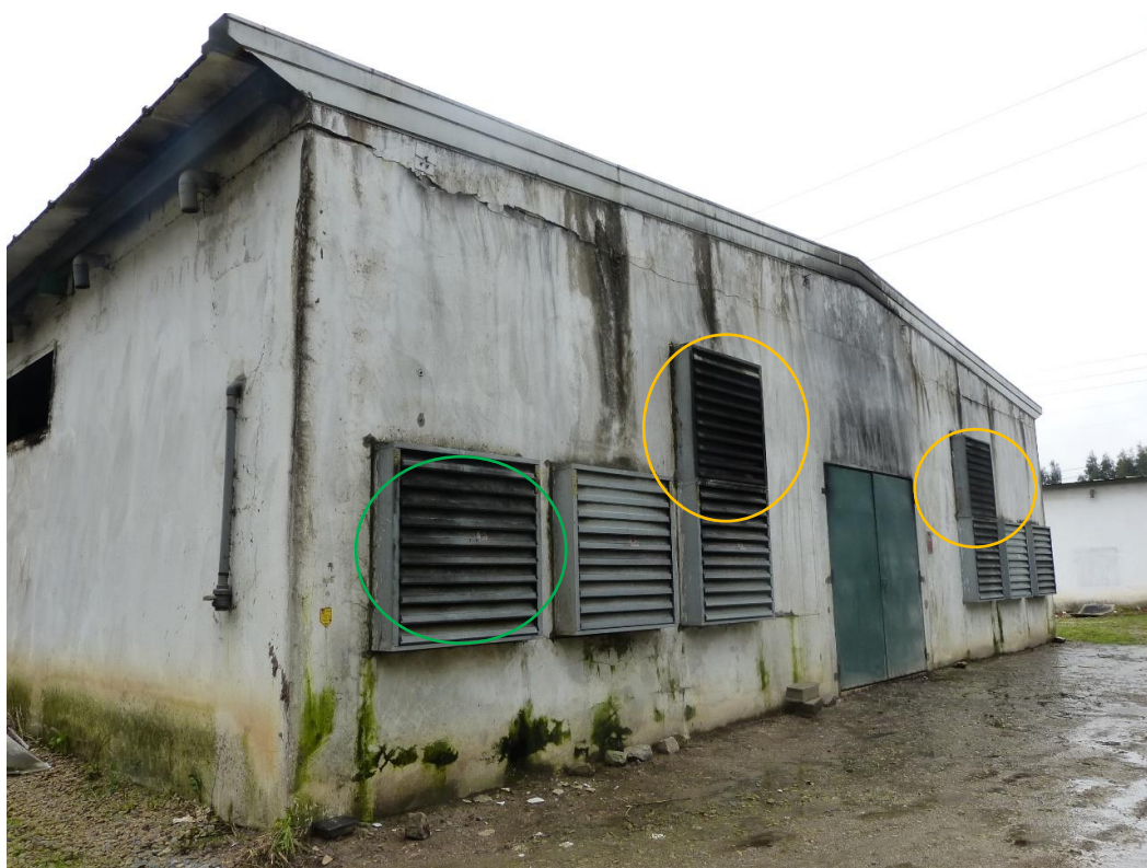
Picture 03 - Outside view of backdoor (north to south) – compared to the front entrance, here there are signs of the fire visible, on top of the main door and on the two top ventilation shafts (orange circles) and on the left one (green circle); darker soot present on the top shafts than the top one, indicating that the smoke and flames were at a high level at the time when they reached the end of the pavilion.
