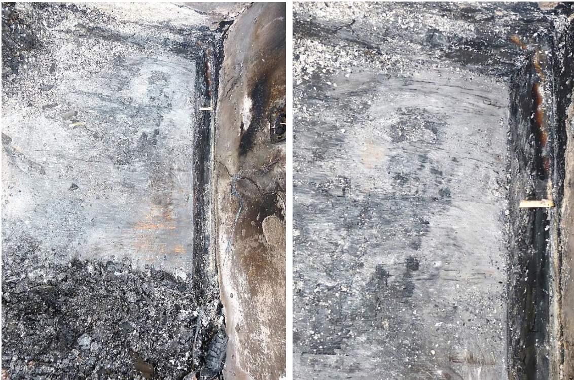
Picture 18 – Detailed view of the floor where the table was located (see previous photos). After removing the debris, there was the absence of any damage to the floor level, which allows us to exclude that a fire started at that point, especially with the use of an ignitable liquid as a fire accelerant.
