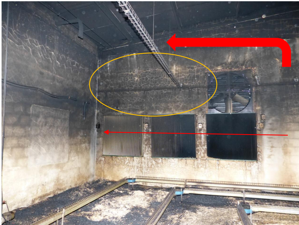
Picture 42 -Corner of west and north walls – alligator marks (orange ellipse), signs of dehydration after a long persistence of high temperatures and smoke; decreased damage from up to down and from right (east) to left (west).
