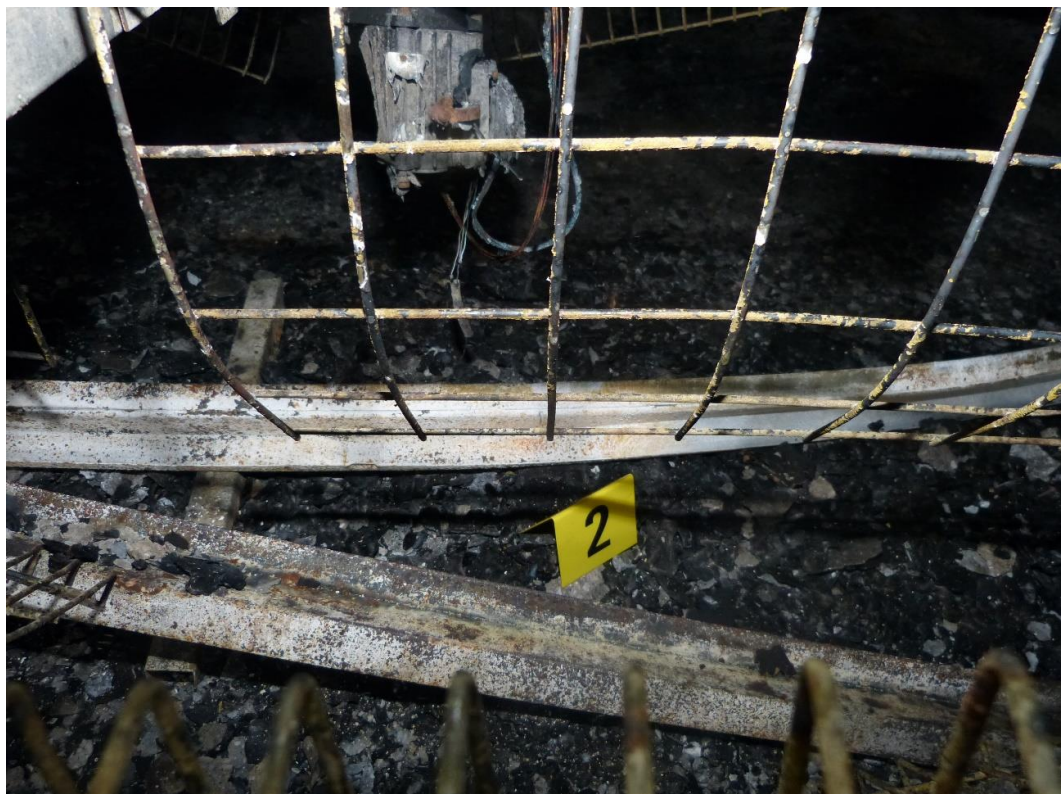
Picture 23 - Tag #2 view from top, east (top) to west (bottom) – high damage area on floor, signs of low level slow burning.
