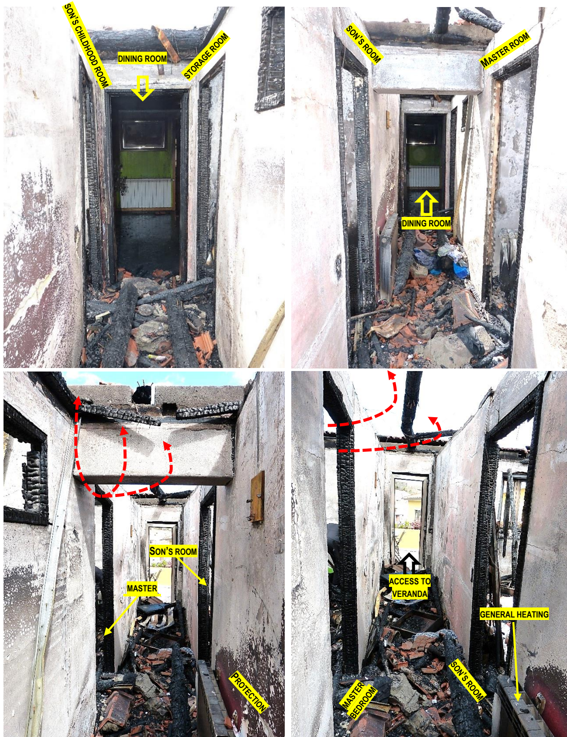
Picture 10 – In the corridor uniformity in the degree of damage is observable, confirming that the heat transfer occurs mainly by the upper area - full destruction of the false ceiling and cover- it is possible to see greater protection areas at a low level with the presence of the original paint on the walls and the preservation of the central heating.
