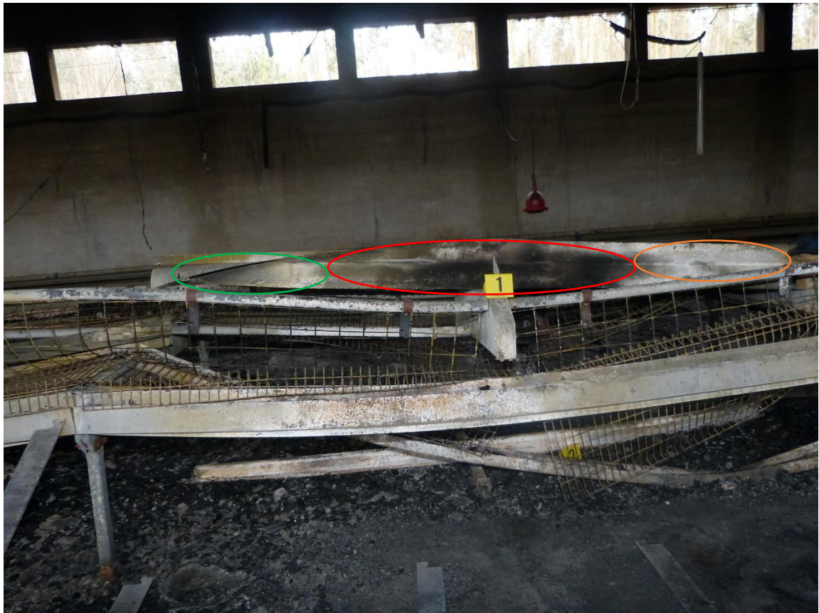
Picture 24 - View from underneath of central metal bar near tag #1 – direct flame contact in black area (red circle); protection on the left side of the metal bar (green ellipse) and exposition signs on the right (orange ellipse).
