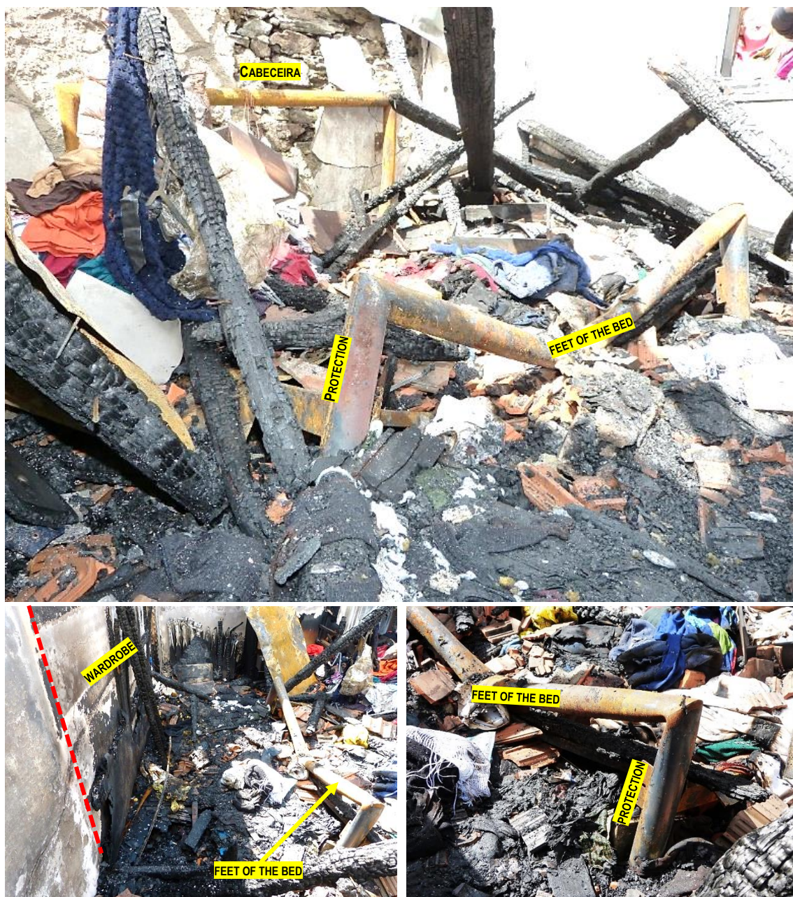
Picture 19 – Perspective of the couple's bed, metal frame, identifying different degrees of damage. In the horizontal bar and the support feet a low degree of oxidation on the face exposed to the wardrobe and the table is observable, confirming their remoteness from the initial point of combustion on the head, where a higher degree of damage is visible.
