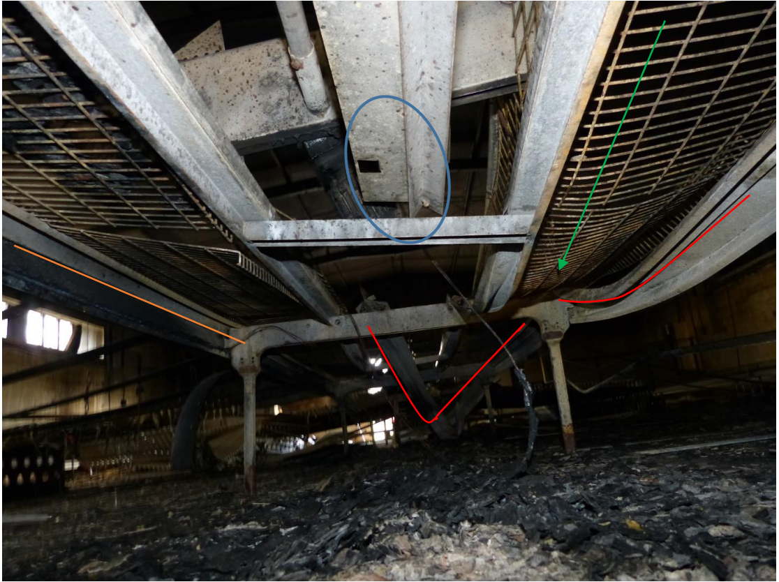
Picture 36 -View of left side of tag #7 from bottom – high deformation of metal bars (red lines) on the right side (west) of the picture compared to the left side (east), indicating propagation direction towards west and not east from the motor (blue ellipse); increased oxidation levels of metal fence towards the motor (green arrow), pointing to the point of origin.
