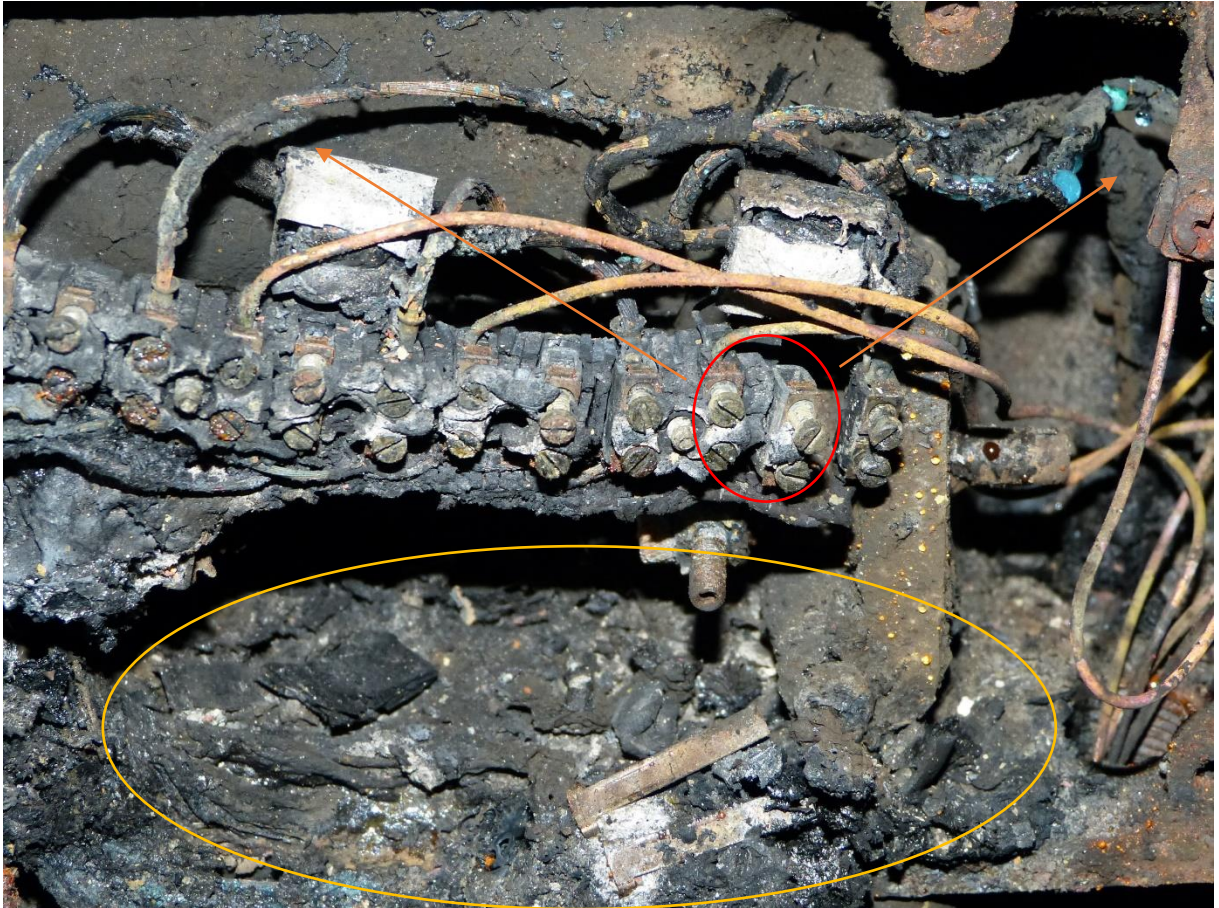
Picture 38 - Close up view of motor (tag#7) – highest degree of damage between 2 nd and 3 rd contact (red circle), from there V-pattern can be observed on the levels of damage; radiant heat damage on the part below the contacts (orange ellipse).
