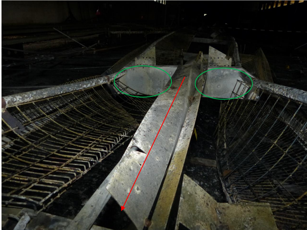
Picture 16 - Tag #2 – view from the left side (north to south) – middle horizontal metal bar is protected from this side (green ellipses) – vertical bar in the middle shows decreasing damage/oxidation from south to north, confirming the direction of propagation of the fire.
