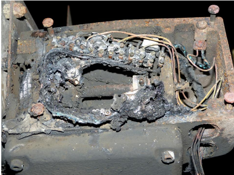
Picture 39 -Close up view of motor (tag#7) II – high oxidation levels on the upper right side but higher damage levels on the lower left side, indicating that the fire started there, but then traveled downwards.
