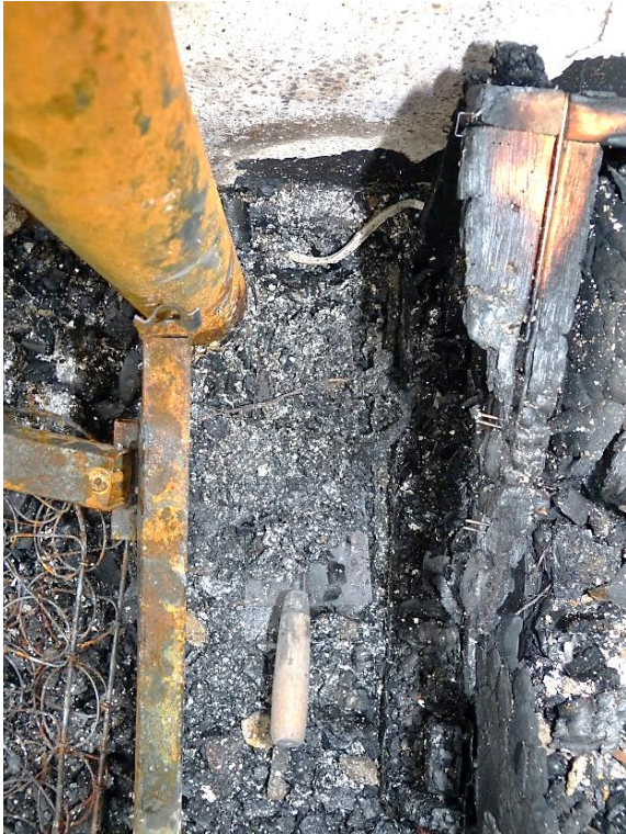
Picture 23 – On the floor between the bed and the bedside table debris of the alarm clock that was originally located on the right side of the table top, coincident with the area of start of fire were recovered.
