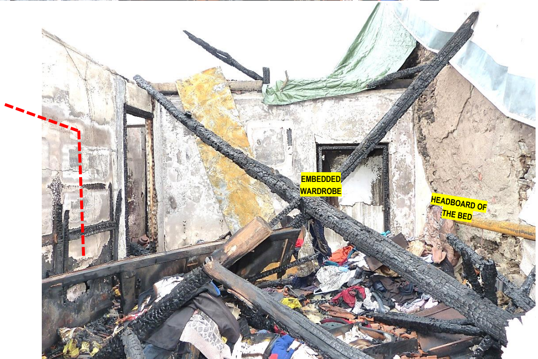
Picture 12 – Overview of the room where the fire started. To be noticed, a greater depth in the degree of damage can be observed, particularly on the wall at the bedside, consistent with proximity to the initial heat source. In the wardrobe leaning against the opposite wall, the damage occurred in the downward direction by the effect of convection currents – red line.
