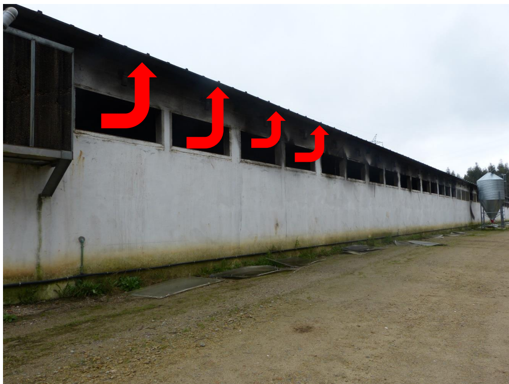
Picture 02 - Outside view of east wall of the pavilion – soot deposition on the top of all window frames, the direction of the flames and smoke coming out of the windows is indicated by the red arrows.
