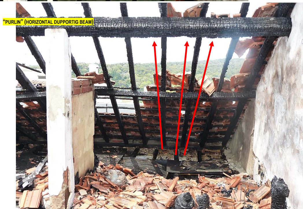
Picture 13 – In detail, seeing that the structures of the "rafters" exhibit charring marks in greater depth close to the "purlin" horizontal support beams- red circle- resulting from longer exposure to the action of heat –red arrows- from a point of origin at a lower level.
