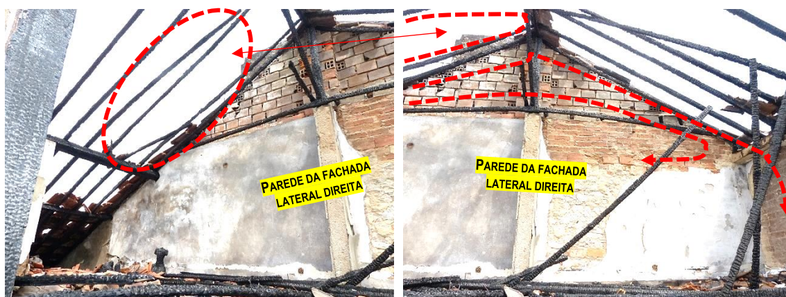
Picture 12 – In the upper area of the room there has been a complete consumption of the false ceiling and an intensive destruction of the coverage (the "Rafters"). This damage is particularly visible in the "Rafters" and "slats" of the structure that exhibit a greater concentration of damage on the front right section of the building –red circle. Also observable are damages resulting from convection currents –in the orientation from the main façade to the back wall, red arrows-, consistent with the direction of propagation from a separate point of origin.
