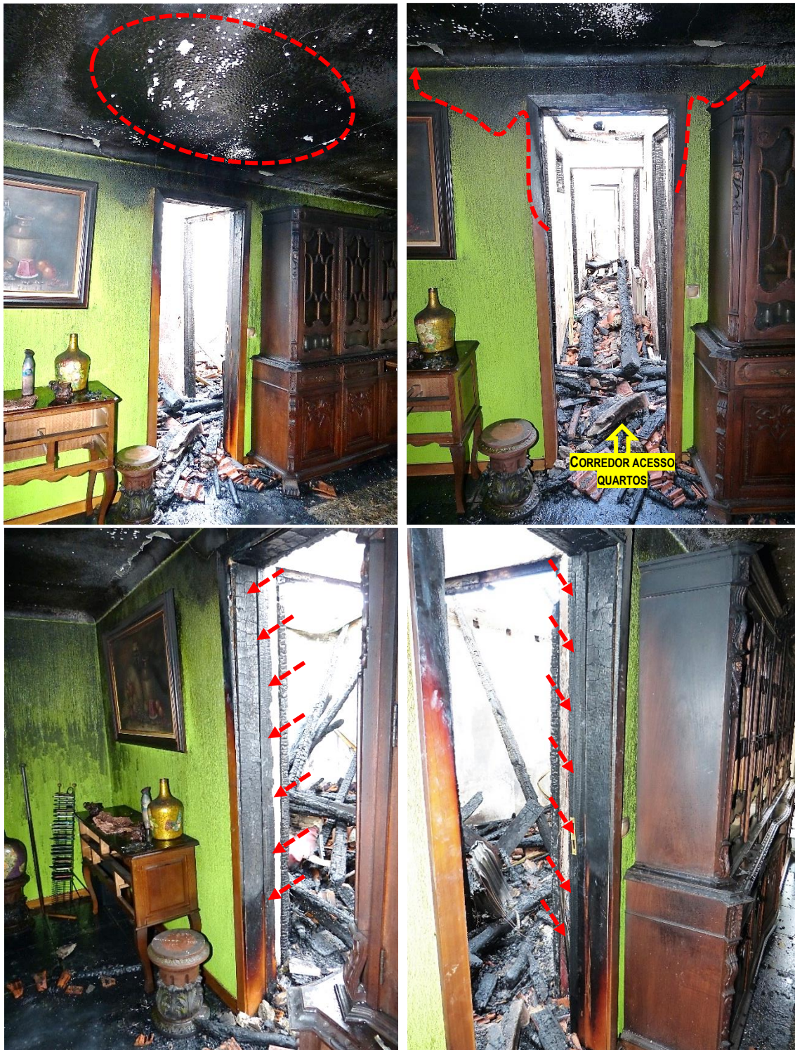
Picture 09 – In detail the damage to the ceiling –red circle - and the door frame of the access door to the corridor to the rooms -which was closed- showing the carbonization of the material downwards in the course of propagation of combustion –red arrows - in consequence of the convection currents.
