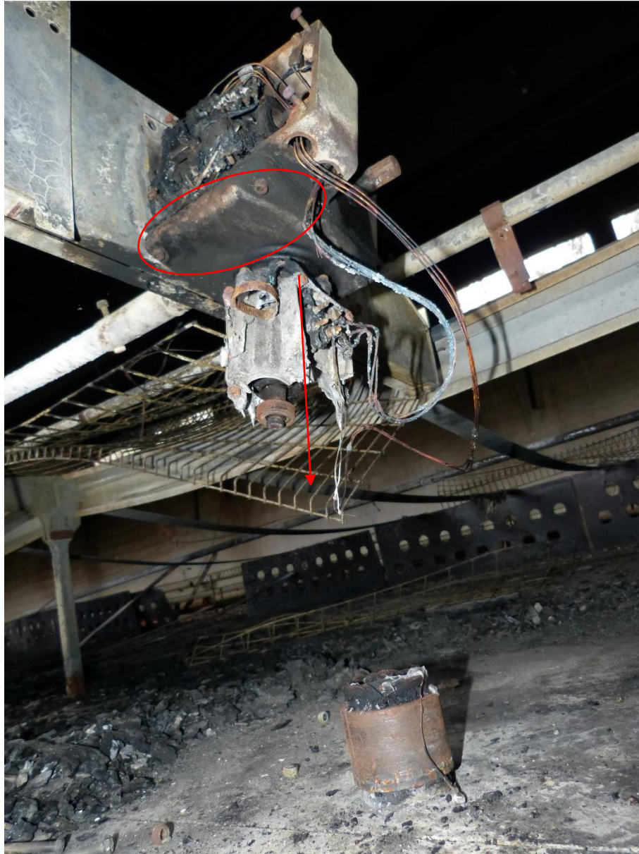
Picture 30 - View of motor (tag#1) from bottom – black area underneath the motor (red ellipse) indicates heat source from underneath; drop-down of plastic underneath the motor (red arrow).
