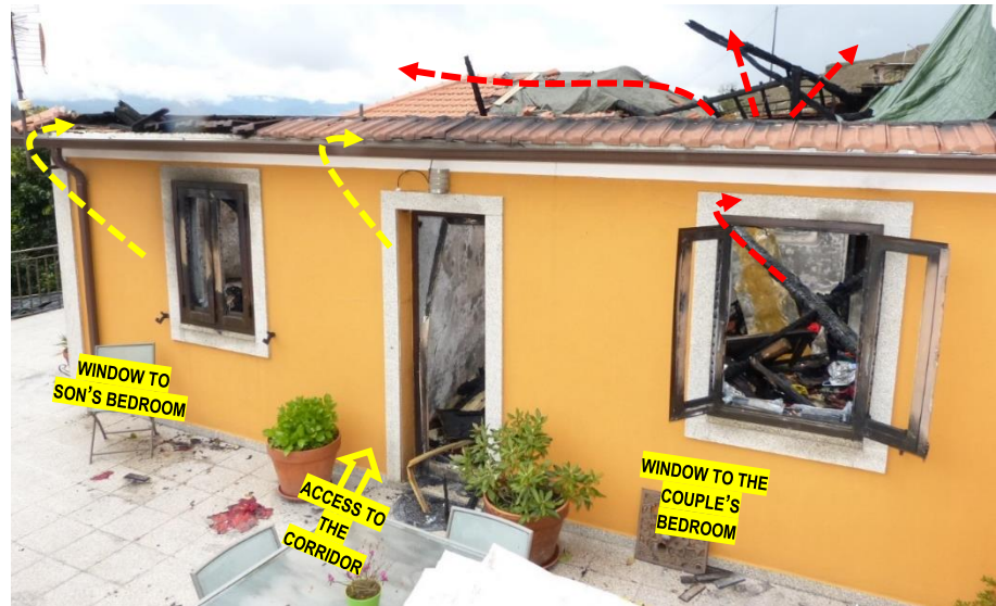
Picture 04 – On the side with access to rooms, two different types of damage are identifiable. In the window of the son's room, as well as the coverage area above a resultant destruction due to a sequential propagation in great amplitude of the available materials –wood and synthetics – is observed, consistent with the distance to the starting point, due to the increased the temperature generated by hot air flows –yellow arrows.
