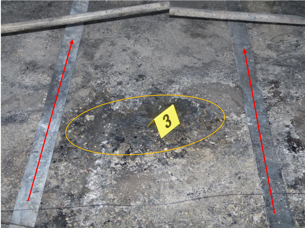
Picture 22 - Tag #3 – detoxification bloc – damage on bars does not coincide with this point as seat of fire, since the damage should have been pointing to the direction of the bloc in a concentric way, but instead the damage is increasing from bottom (west) to top (east).
