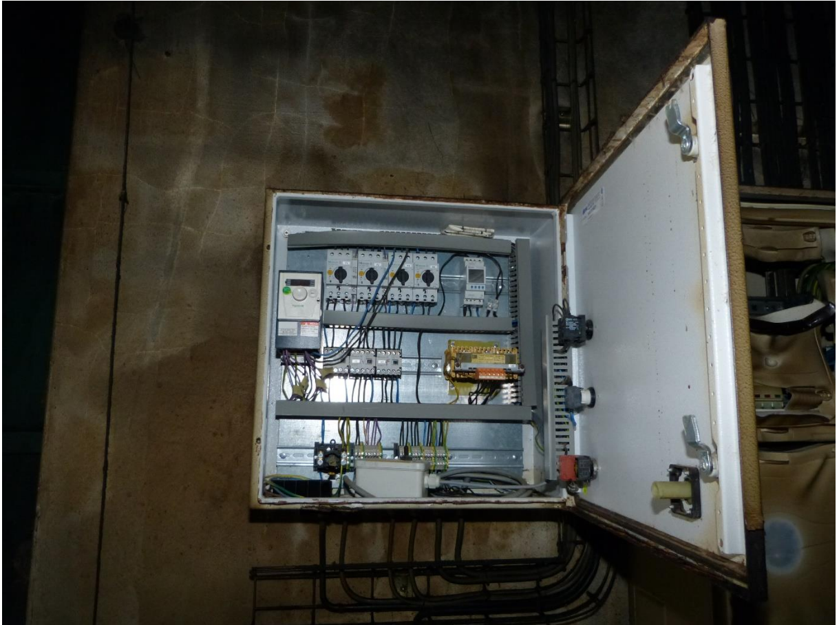
Picture 47 - Electrical box 2 – timer.
