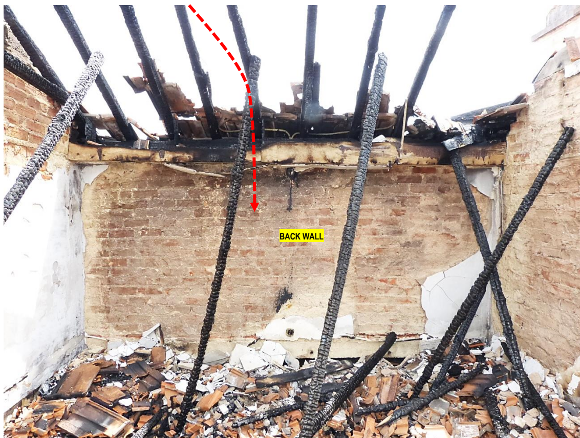
Picture 11 – View of the back wall showing damages in amplitude starting from a higher level, consistent with the reception of heat during an advanced stage of the combustion, in which the fire was already in propagation – red arrows – resulting from the development of a fire originating on the opposite side – main facade.
