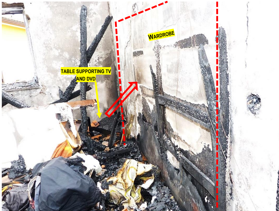
Picture 13 – Observing the heat transfer along the wall where the closet is located, a degree of atypical damage is seen, with a higher degree of carbonization on the left side and starting from a low level, as well as a damage in "V"-shape, resulting from heat received by radiation from the combustion of table, which was covered with a cloth, that supported the TV and DVD –secondary fire-.
