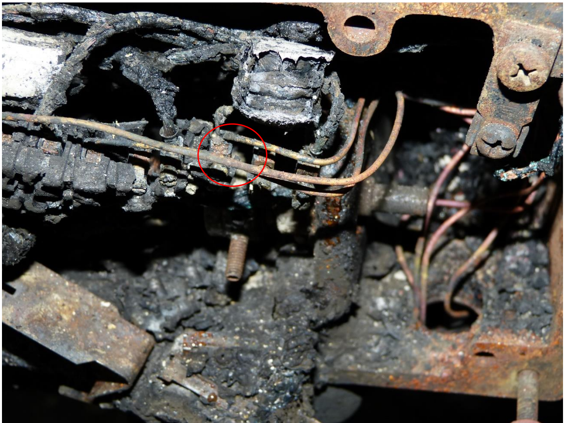
Picture 31 - Close up view of motor (tag#1) from top – point of origin (red circle).
