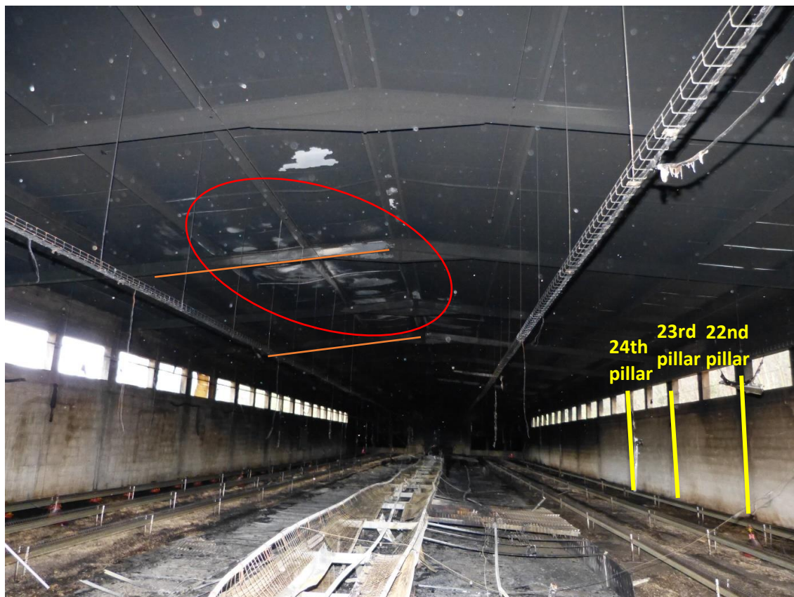
Picture 43 - View of rear part of pavilion – damage on ceiling (red circle) coincides with a direct flame contact for a longer period of time, which is due to the presence of curtains in those points (orange lines), which worked as a barrier for the fire, until the curtain was melted and the fire could 'carry on'.
