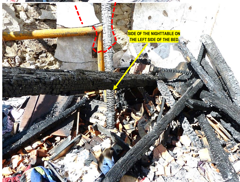
Picture 21 – Headboard. High degree of damage along the whole length of the wall above the bed, particularly on the left side, where the destruction of the plaster denotes an area of greatest and heterogeneous damage, consistent with the position of the bedside table in line with the incidence of a direct source of heat for a longer time period.
