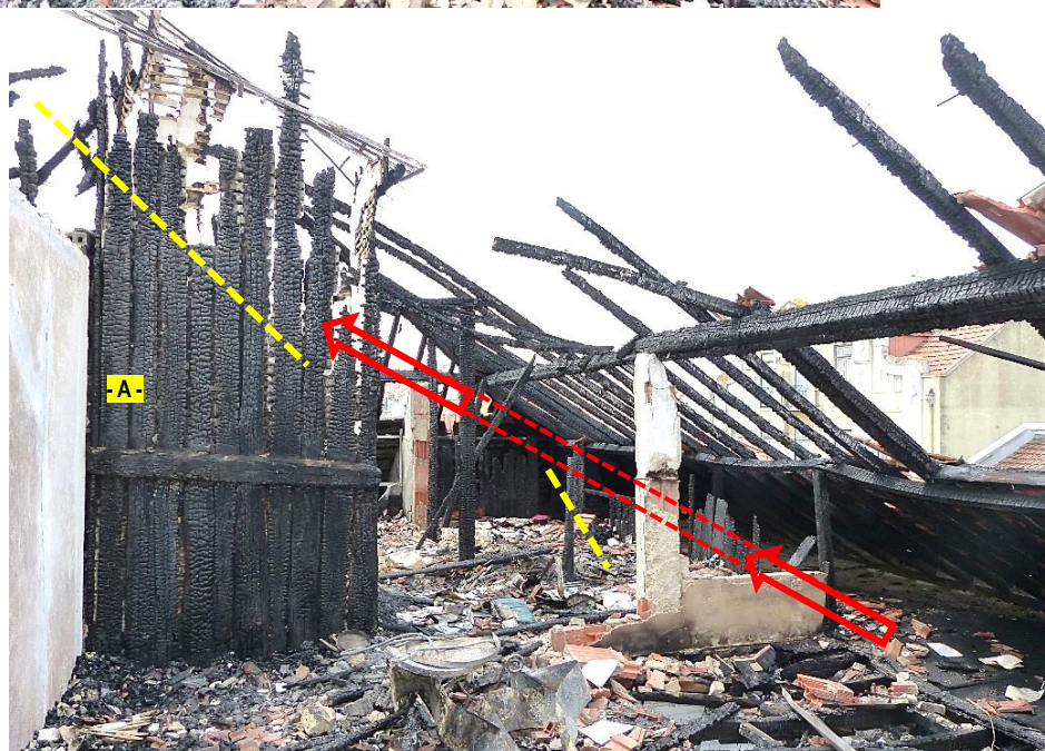
Picture 15 – Perspective of the remaining area. In the structure of the stairwell-box "A" and the masonry pillar damage in a "V"-pattern can be observed, which results from the exposure to direct action of heat transmitted by radiation for an extended period of time from a second point of origin –tag #2 - present on the right side –red arrow-, on the main facade and one level below the window - B -.
