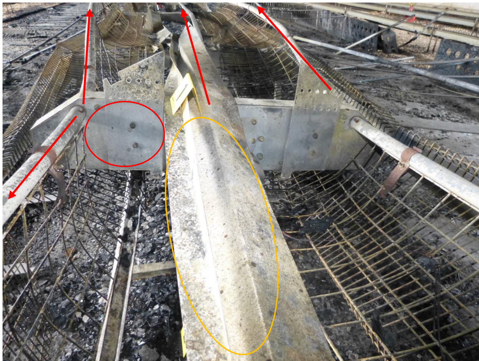
Picture 15 - Tag #1 – View from the top, south to north – damage decrease from north to south (orange ellipse), side is clear (red circle), indication of direct flame contact for a prolonged time, while the other side is protected; red arrows show direction of propagation.
