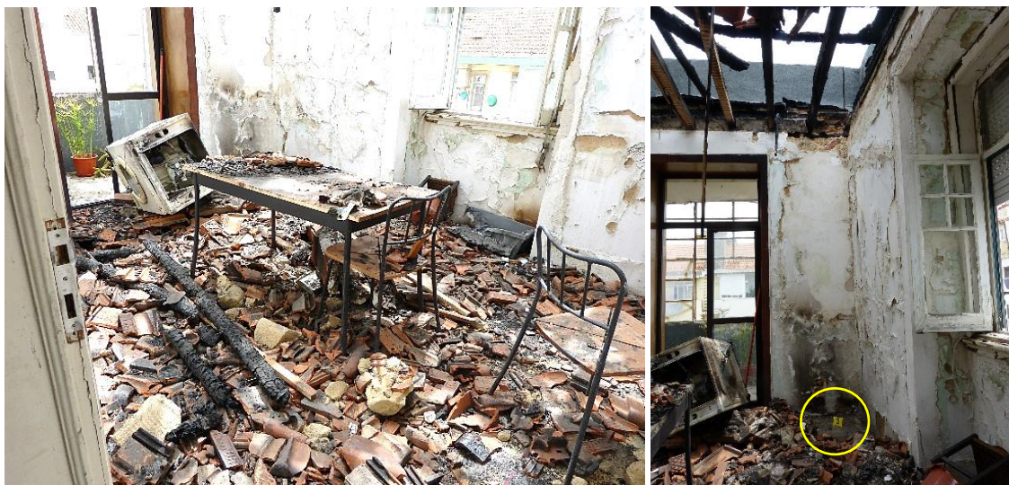
Picture 05 – Inside of the dining room, observing a degree of complete destruction of the ceiling and the main wooden structure between the floors. Accordingly, it appears that the lower face is protected, consistent with heat acting downwards from an upper level, the attic. This damage is particularly visible at the corner, where it is limited and the degree of carbonization of the structures is higher, resulting from its proximity to a circular point of origin – red circle. Yellow circle indicates tag#3, where a sample was collected for laboratory analysis.
