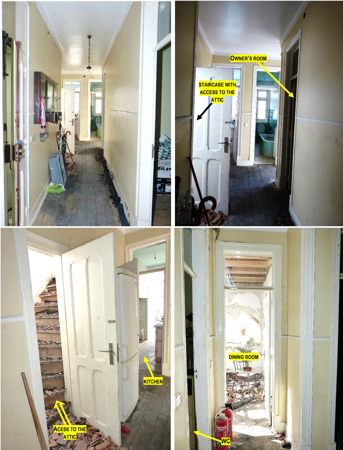
Picture 04 – View of the apartment’s entrance hall, where it is observed that there is no damage from the spread of fire, except at the level of the area in the living room corresponding to the damaged area in the attic, which resulted from collapse of the false ceiling, indicating the development of the fire from the top floor -attic-.
