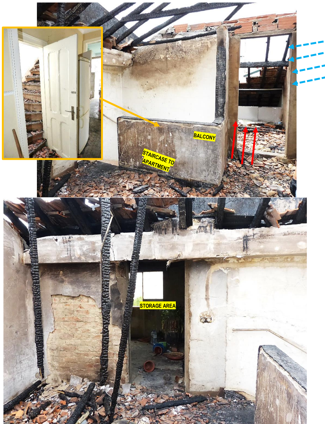
Picture 07 – Area of the attic with access to the stairs to the apartment. Especially on the balcony damage indicators of both directions of propagation are visible, meaning they originate from opposite points.
