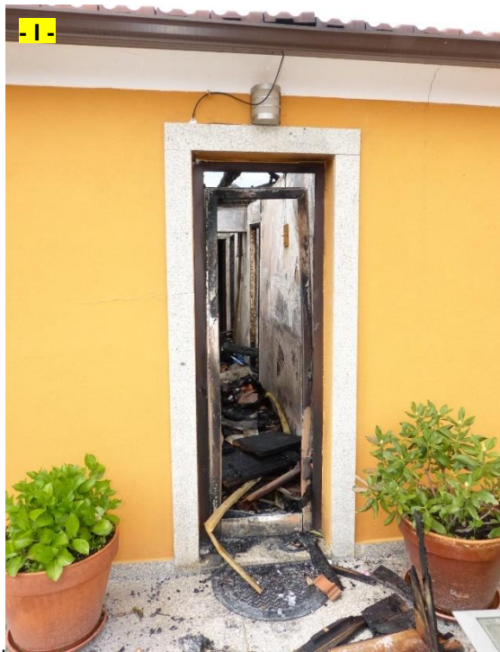
Picture 05 – In detail the contrast between the destruction observed along the front window of the son's (-II-) and couple's (-III-) bedroom, identifying a sense of clear spread in the latter resulting from a combustion point located at a lower level on the right side –red arrow. On the contrary, in the corridor area and the son's bedroom window, the marks are the result of a heat accumulation in downward direction and in greater range, consistent with a fire already spreading.
