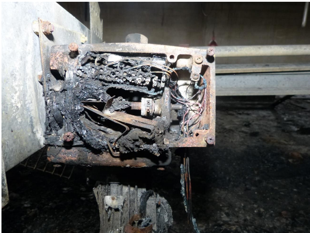
Picture 25 - Damage of motor (tag #1) from front.
