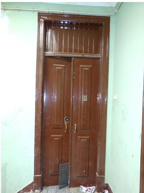
Picture 02 – Main door of the damaged apartment – outside view.
