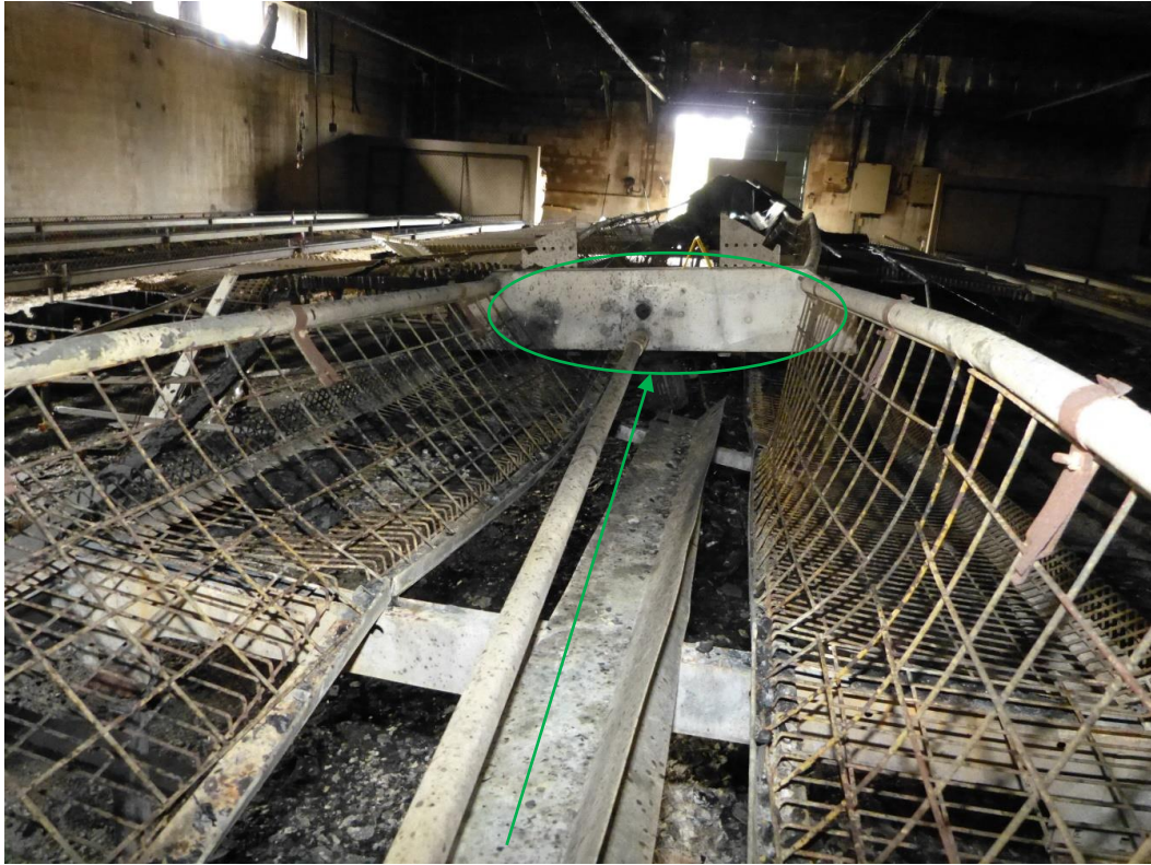
Picture 34 - Tag #7, view from left side (north to south) – increased oxidation level from north to south (green arrow), protected left side of metal bar on left of tag#7 (green ellipse).
