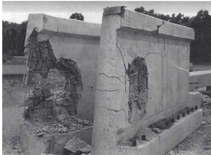
Figure 2.11: Reinforced concrete after EFP impact [52].
