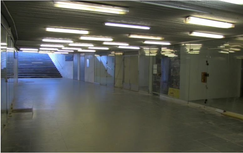
Figure 2. The decaying underpass under the ground
